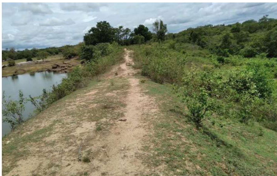
Figure 2-7 Vegetation grown on the tank bund to be removed (7°34'50.7"N 81°35'50.6"E)
